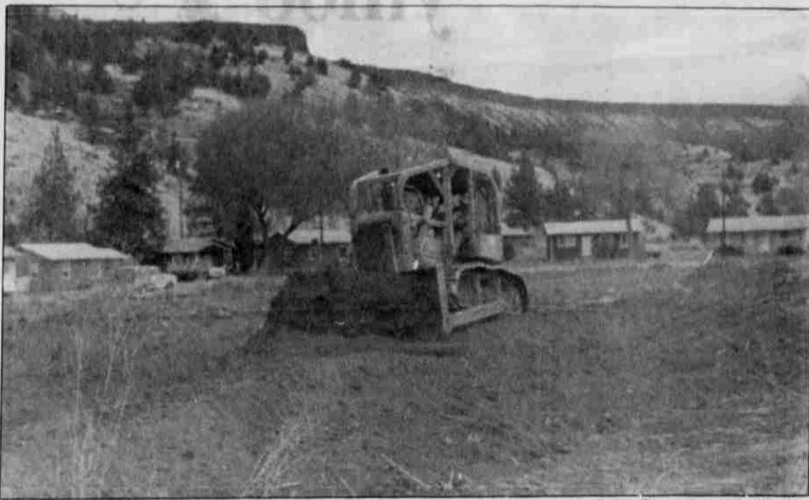
Spilyay Tymoo photo by Bob Medina. Heavy equipment has been busy at the site of the Museum Village Retail Center, due to open later this year.
