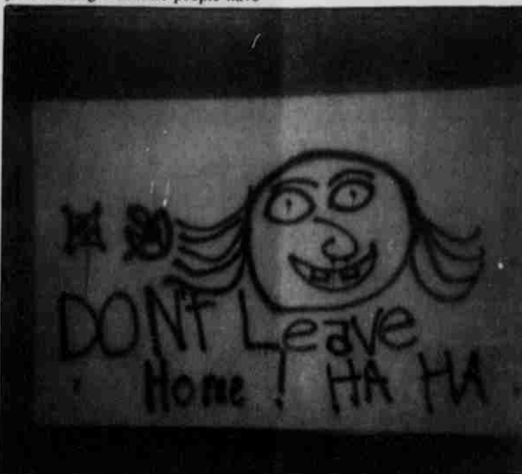
Black spray paint was used on wall of new home by vandals.
