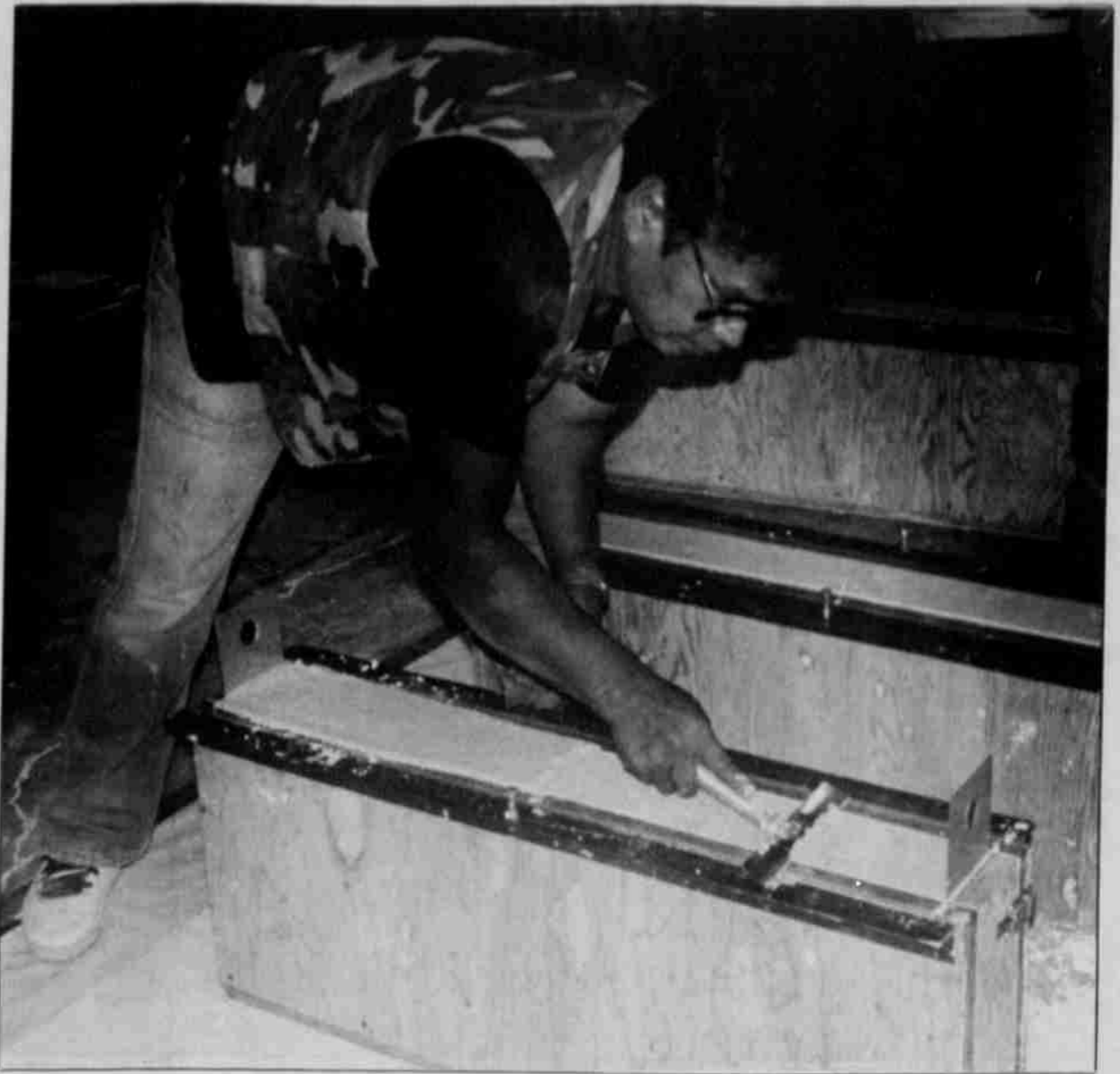
Louie Tewee works gelatinous material after it has been poured into brick mold.
