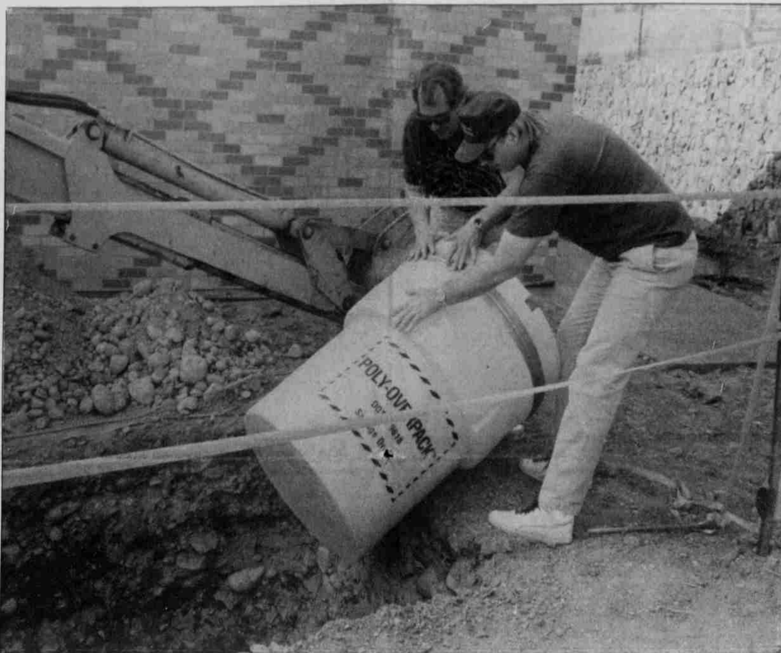
Museum construction workers drop time capsule into ground at new museum site. Capsule will be opened in 100 years.
