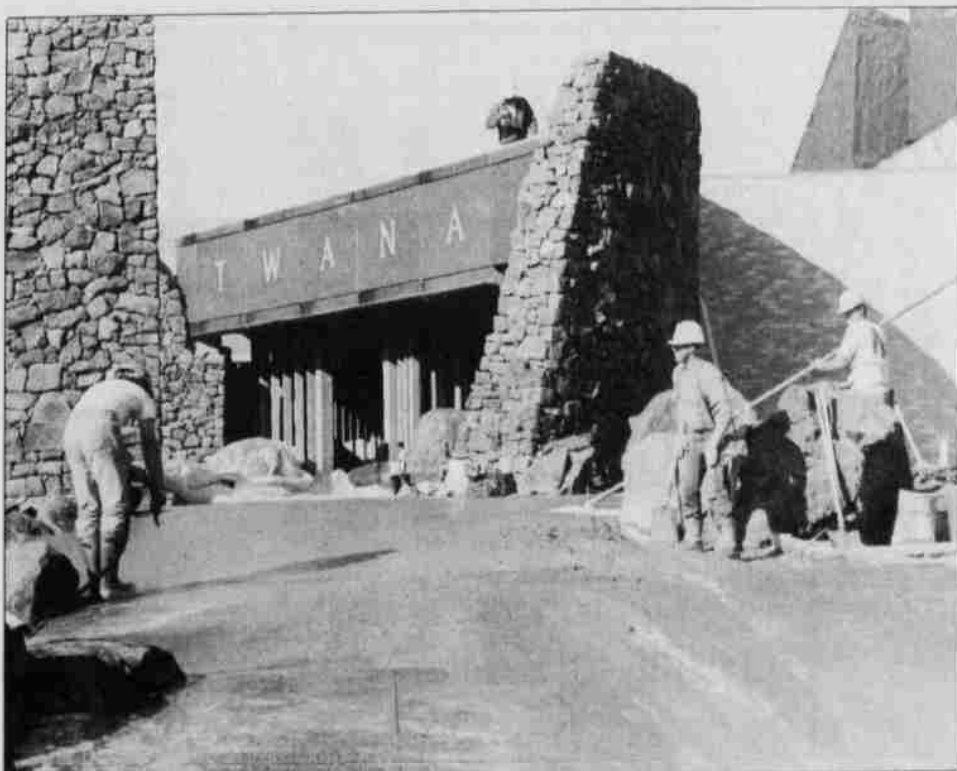
Work continues on the Warm Springs Tribal Museum. Completion date is set for early 1993.
