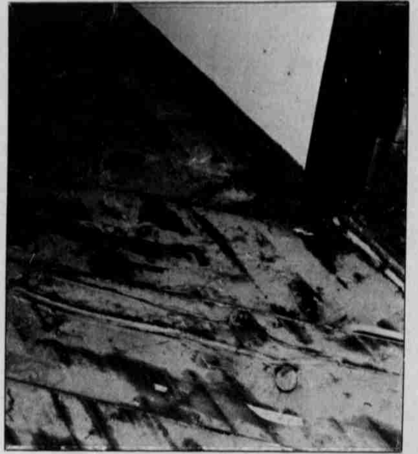
Damage done to floor located at the Warm Springs Fire and Safety office was caused by termites.
