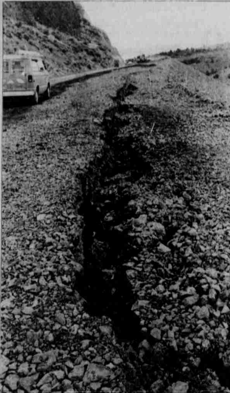
Slip slidin' away—After nearly four months of work on the grade south of Warm Springs, an ancient slide was reactivated. The slide has caused new fill material to break away and fall into the canyon. State highway officials are not yet sure how the slide will be handled.
