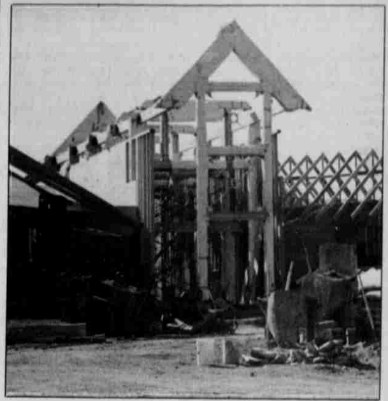
Offices for Warm Springs Power Enterprise is nearing completion. Plans call for occupancy by fall 1990.
