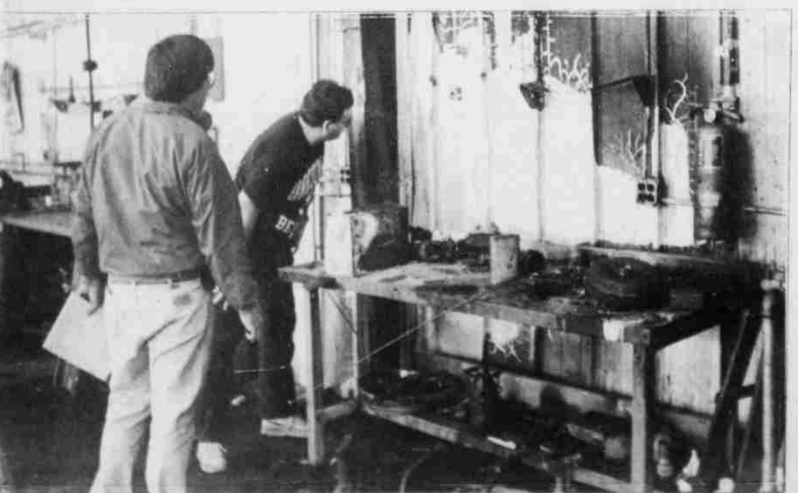
Jerry Huff and Dean Seyler viewed the damage to garage walls and work space the day following the fire. Estimated damage has been set at $3,000.
