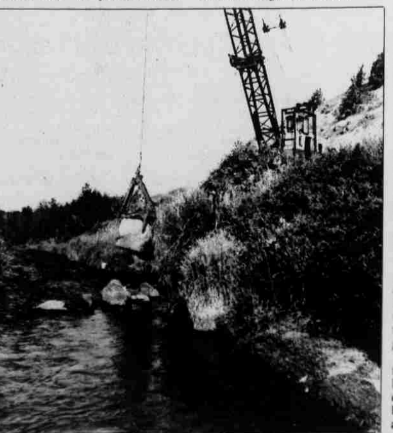
WSFPI and Warm Springs Natural Resources department worked together to protect the aquatic ecosystem of a small diversion channel.
