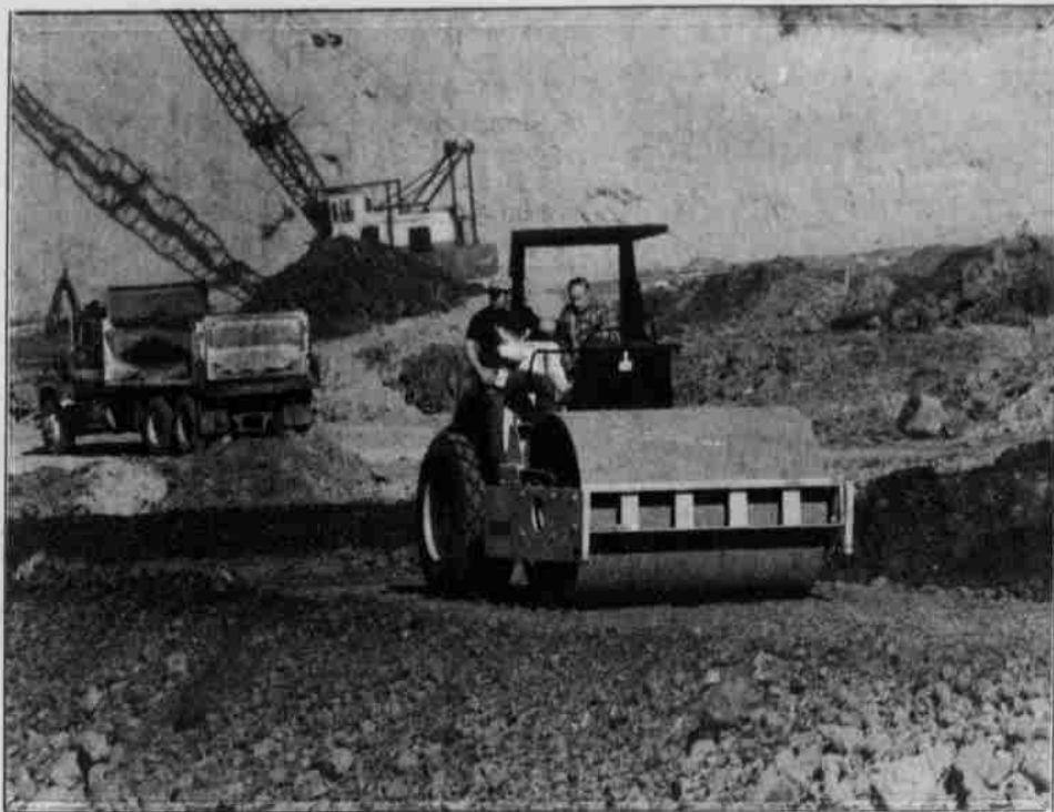
While a roller and dump truck prepare the yard for future construction, a shovel, in the background, continued to unload log trucks.
