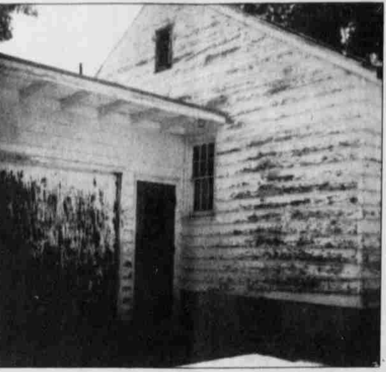
House #2122 on Warm Springs Street was in bad need of a fresh coat of paint recently. Community Service Workers were detailed to sand blast the house. They followed with fresh white paint and blue trim.
