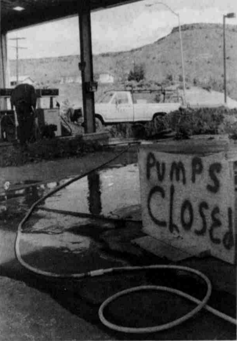
The concrete covering the fuel lines leading to the pumps at the garage has been removed since this photo was taken. The removal was necessary so that the lines could be accurately pressure tested.
