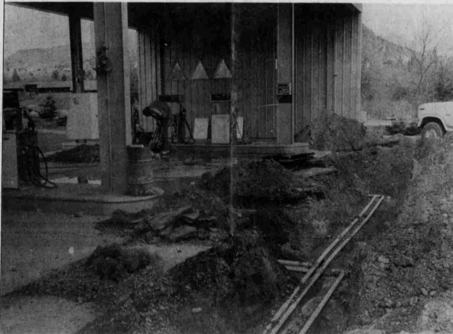
The fuel pipes and tanks at the Warm Springs tribal garage were unearthed after the discovery of a fuel leak in the lines. The garages continues to service vehicles, but is no longer pumping gas. It is unknown when the garage will resume pumping.
