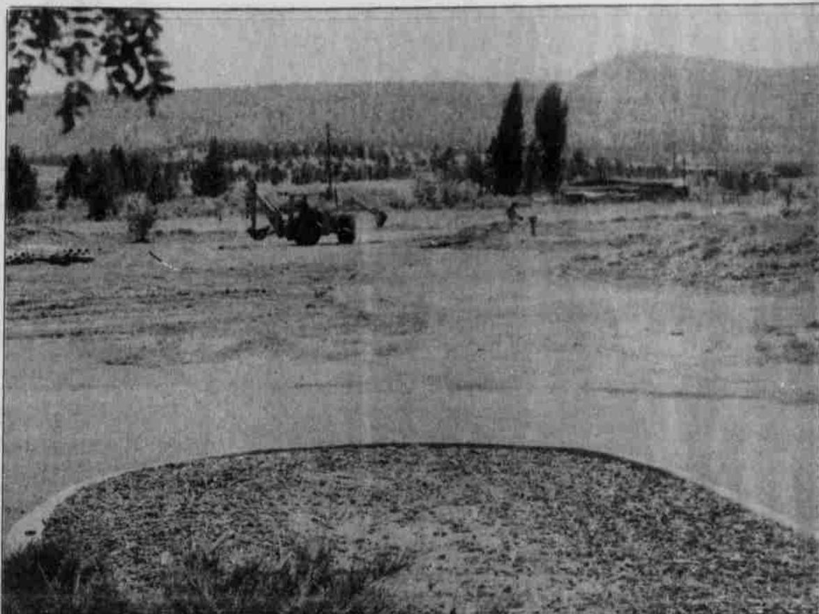
Work started on the construction of the new housing office for the Local Housing Authority (LHA) which will be located just southwest of the Administration Building. Crews prepared the site and on August 26, crews began pouring the footings for the foundations, according to Bill Caudle, tribal construction manager. The project is scheduled for completion January 1.
