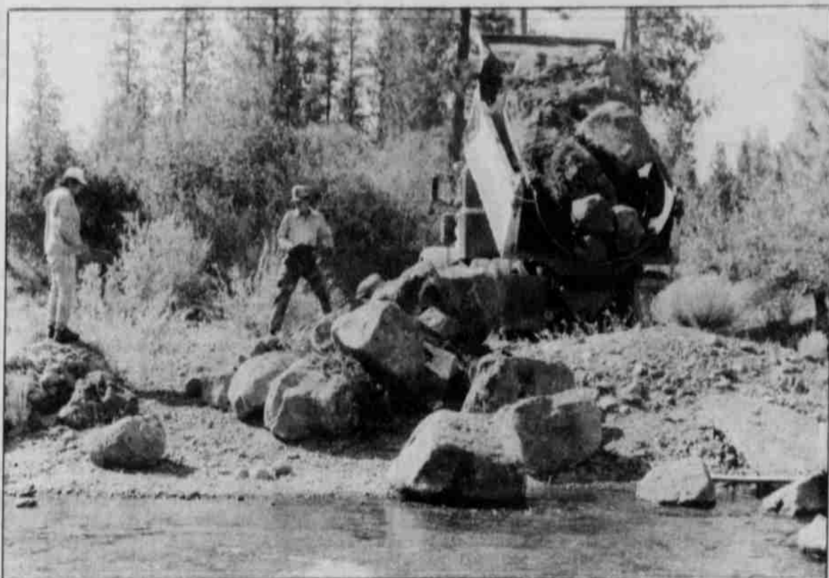
Rock placement begins Rehabilitation work on Mill Creek at Potter's Pond has begun. Seven hundred boulders will be placed in the stream providing pools for migrating chinook and summer steelhead.
