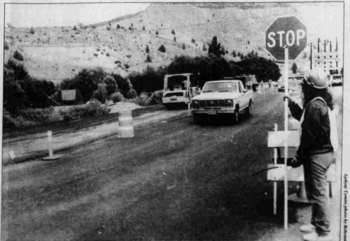
Work on the Deschutes River bridge has tied up traffic for short periods of time. Traffic stops will probably cease next week.
