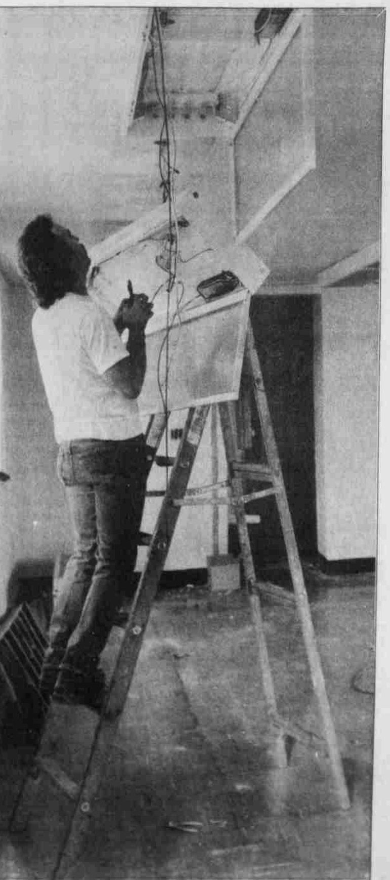
Brad Goldrick works at removing old light fixtures to make way for drop ceilings in the old administration building. Renovation of the building began in late January and is due to be completed in April.
