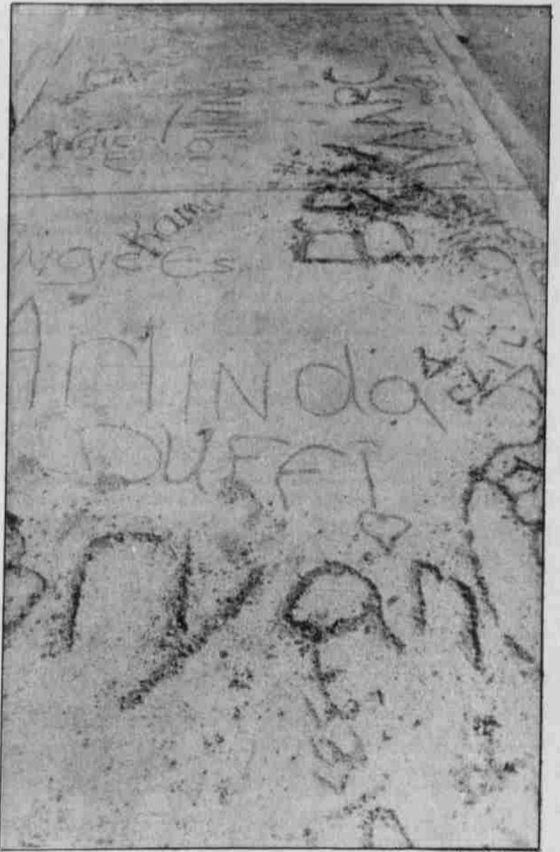
Public sidewalk, vandalized by Madras Jr. High students, had to be replaced. Many of the names written in the cement were put there by other students.
