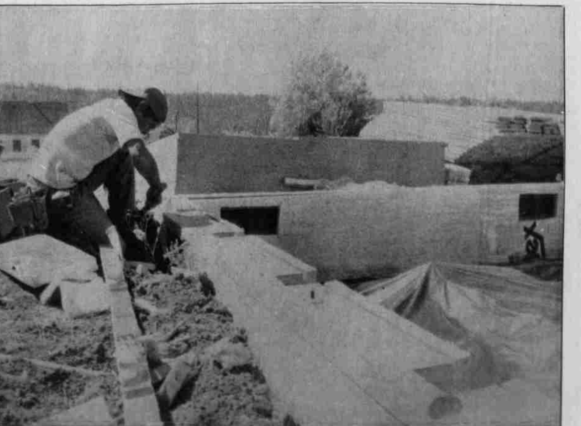
Charley Market in Simnasho is taking shape quickly. Logs are soon to be stacked to form walls for the building. Opening day is scheduled for Thanksgiving weekend.
