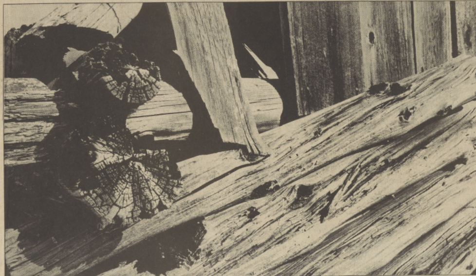
Time has taken its toll on log structure once used as shed at old Dan Howard homestead near Red Lake.
