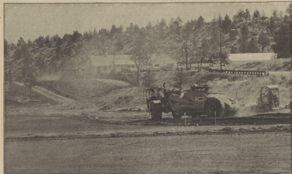
Work has begun on East Tenino road. Eventually the road should extend further down Shitike Creek and enter Highway 26. For the present it will give a new access to the tribal utilities and construction departments.
