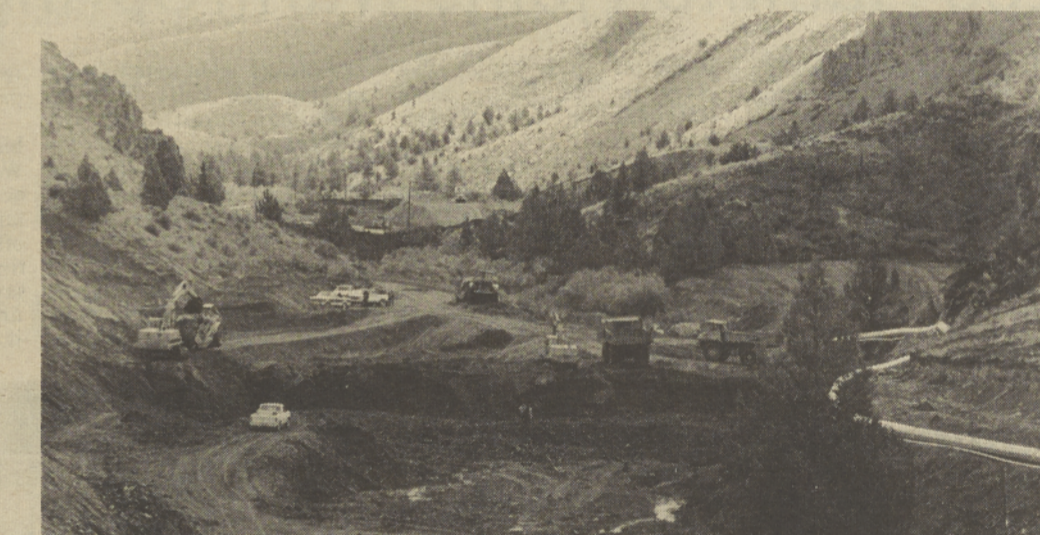
Construction of a dam to provide water for the irrigation of 400 acres is underway. A small hydroelectric plant will be built upon completion of the dam.
