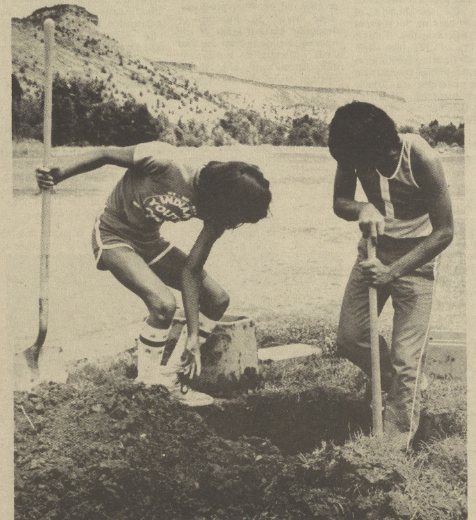
Digging holes is a task that takes both time and energy. David Lucei (right) and Steven Andersen worked throughout the summer on the Community Center water system.
