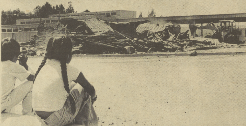
A FRONT ROW SEAT —Shawn Culps and Stacey Squiemphen had the best seats in the area to watch heavy equipment push the old tribal garage into a pile of rubble to make way for the new parking lot for the brand new garage.
