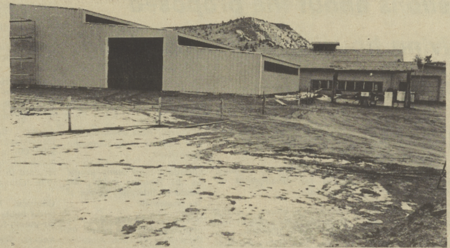
Work on a much needed enlarged tribal garage complex was begun in 1981
