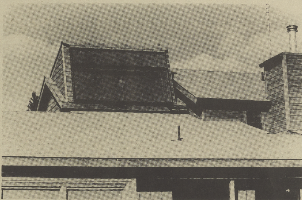
Solar panels collect heat to warm this Warm Springs home's water
