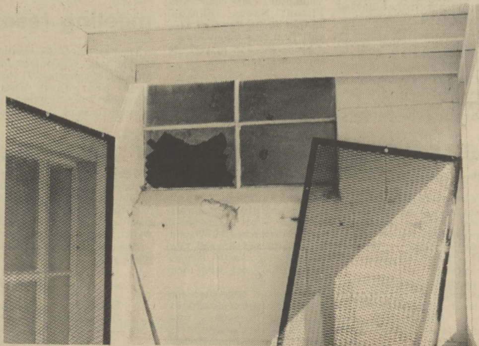
SENSELESS —Motorcycle-riding vandals entered the Shaker Church September 17 through the above window after tearing off the heavy screens. Wooden crosses were strewn on the floor, several other windows were broken and fixtures damaged. Repair costs to the tribes are estimated at about $1,000. Nearly $77,000 had just been spent to renovate the church.
