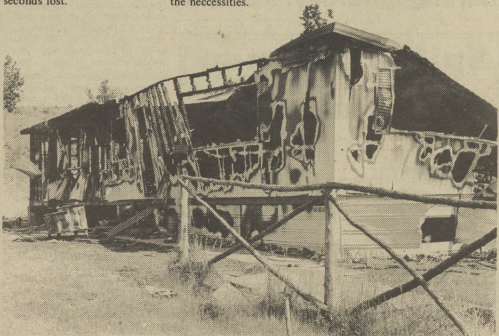
RAVAGED — Fire totally destroyed the mobile home of Versa and Snuffy Smith Saturday afternoon, May 31. No one was injured in the blaze which was most probably caused by an electrical malfunction. A 15-20 MPH wind fanned the flames, hampering the efforts of firemen.
