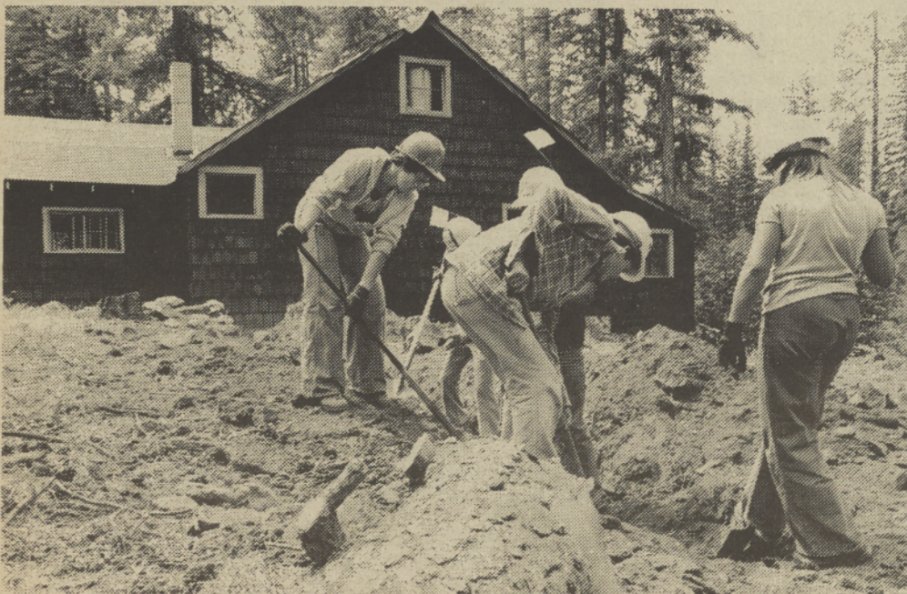
CHECKING THE SEWER LINE - YCC crews have been busy evicting rats and bats from the attic of the Schoolie Ranger Station and performing general clean-up duties in preparation for the Tribes' Wilderness Program scheduled to begin August 1. The workers even located the sewer line and dug it up by hand. Spillyay Tymoo Photo by Rangila
