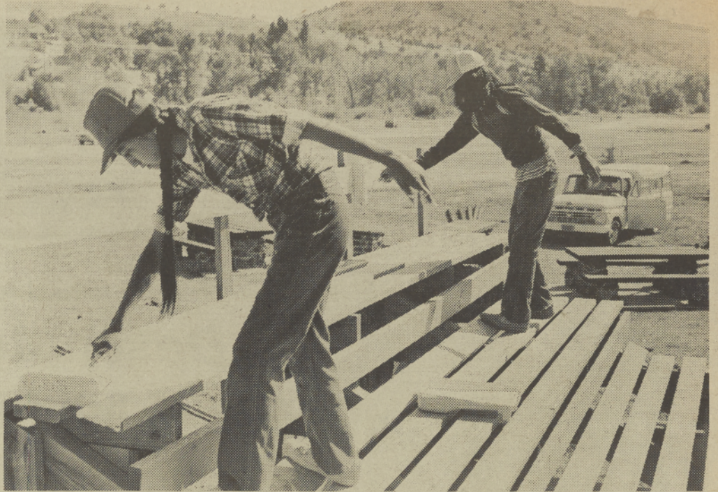
Aldwin Keo, left, and Joseph Winishut gave the bleachers at the Community Center a fresh coat of paint last week. They are with the Field Projects crew of the summer work program for returning high school students. Sixteen workers and two leaders, Eliza Hicks and Brenda Scott, make up this crew that does general maintenance work around the area. Summer workers earn $2.90 per hour and work a 40-hour week.
