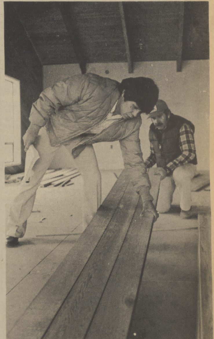
INSPECTOR - Clerk of the works trainee Alvis Smith, Jr., inspects construction sites to make sure contracts are being carried out properly. He checked the paneling for the senior citizens community building recently. Spilyay Photo by CDS
