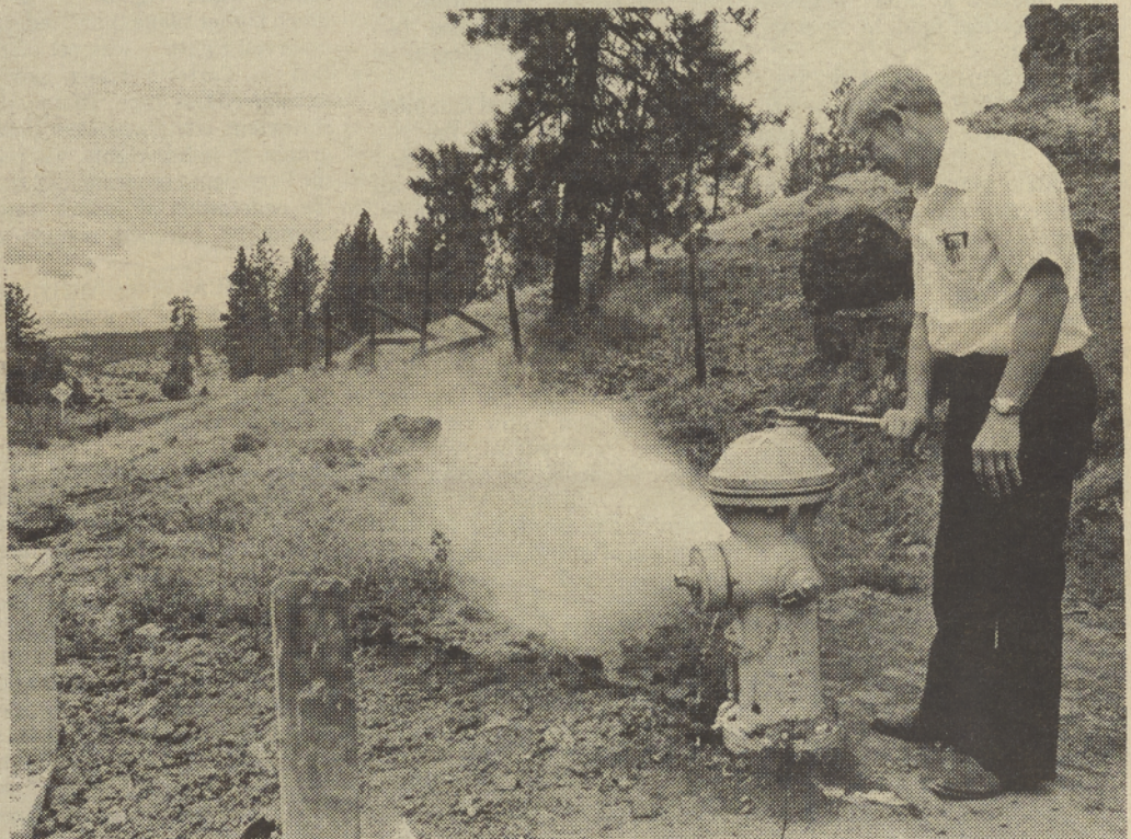
Project engineer Don Rohde of Tenneson Engineering checked one of the eight fire hydrants included in the new water system prior to the preliminary inspection last week. There were no fire hydrants on the old water system. Sandy Rangila Photo
