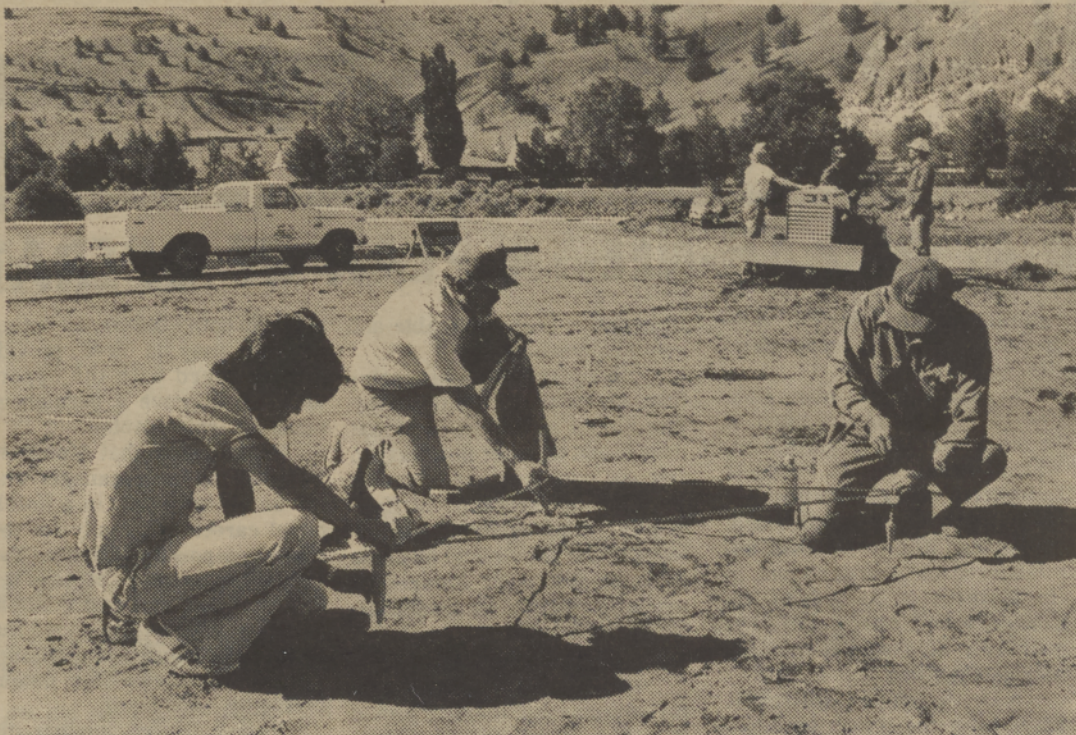
STAKE OUT - Eddie Manion, Dick Souers and Felix Aripa of the B.I.A. Roads Department made measurements for the irrigation system at Kah-nee-Ta's day use area, now under construction. Souers and Clerk of the Works Bill Bennett are engineering the project for the Tribes and eyeing a tentative completion date of early September. The project includes parking, controlled access to the Village and increased recreational area for day visitors. CDS Photo.
