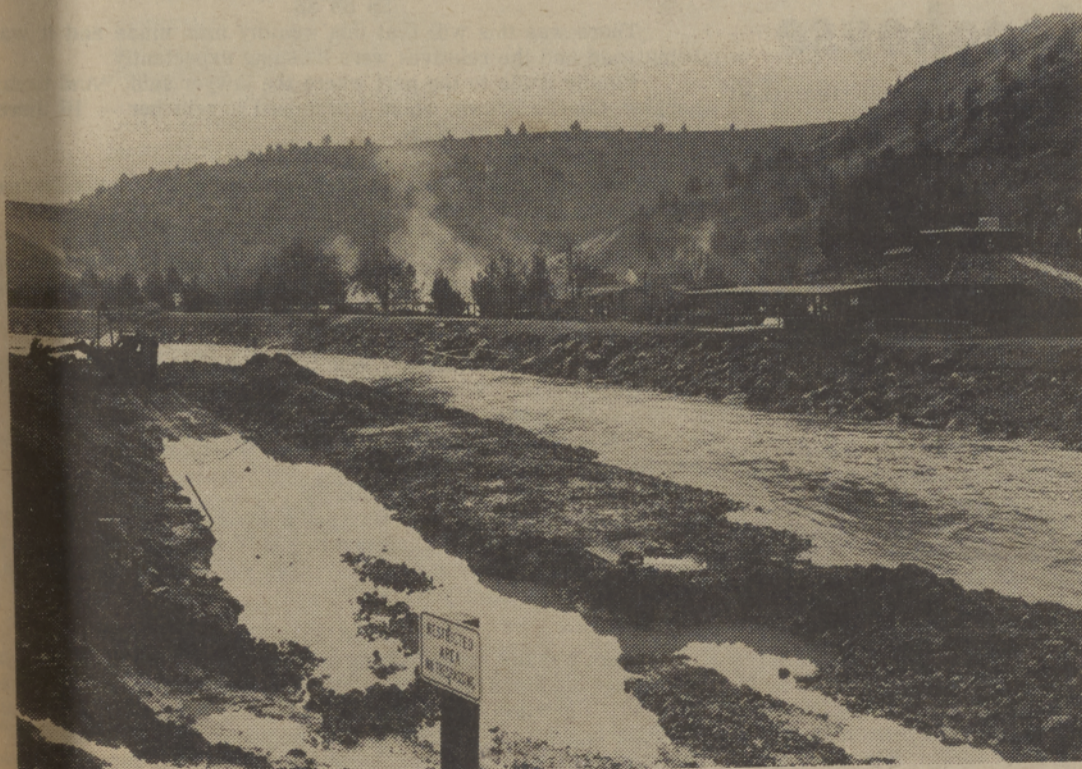
Rip-rapping, or building up the banks with rock, is almost complete on the Warm Springs River at Kah-Nee-Ta Village. The water filtration system, damaged in December flooding, has been repaired but it will take awhile for the water to clear up. CDS Photo
