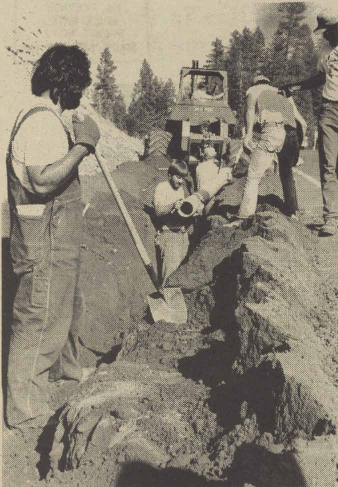
Work began on the Simnasho-Schoolie Flat water project October 17. Workers have laid several miles of 6 inch pipe from Beaver Creek to Simnasho where one of the 100,000 gallon reservoirs will be constructed. (Sandy Rangila Photo.)
