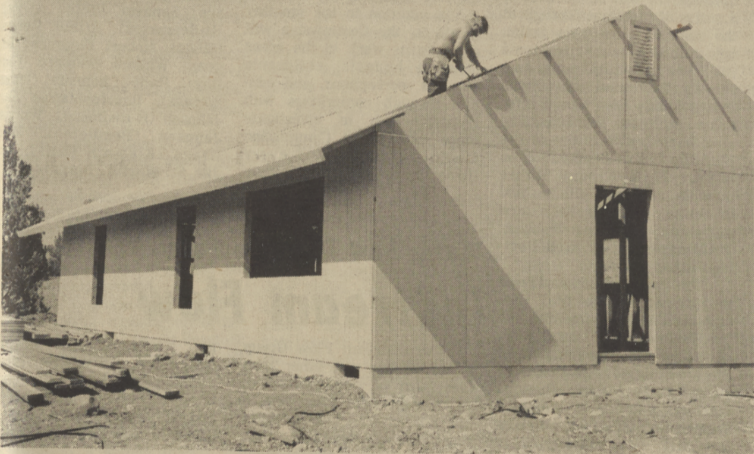
The 30 three and four-bedroom family homes under construction in West Hills are coming along pretty well now. Senior Citizens stopped
