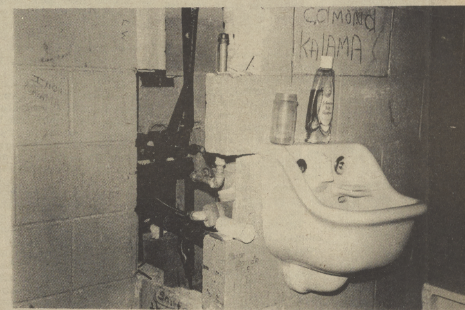
In the women's cell mortar has been dug out with fingers and the brick removed and broken up. A rough-edged pipe sticks out from the plumbing creating a hazard. Neither the structural materials used in the cell nor the sanitation facilities meet jail standards.
