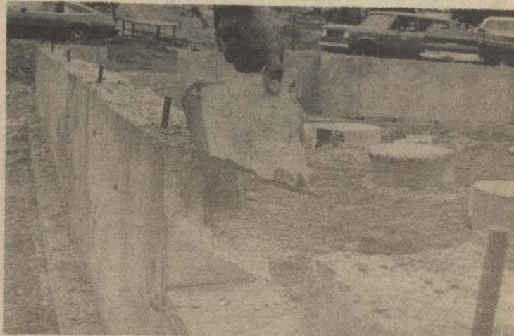
Poor workmanship on the cement foundations forced a halt to construction on the senior citizens units on Elliott Heights June 16th. The problem is being corrected. (Sandy Rangila photo)
