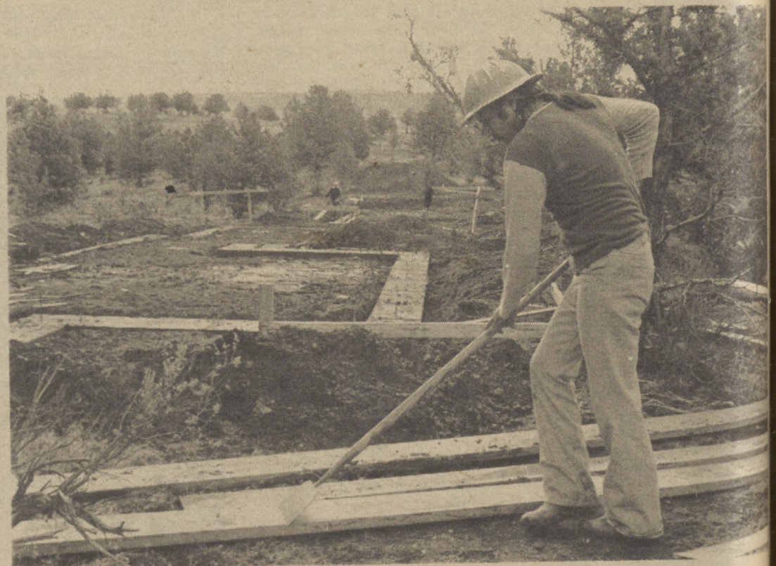
Construction on the tribal apartments began May 2 and by May 11 there were visible hints of the townhouse-style structures. Willie Stacona cleans boards used to make fittings (background) on the construction site south of the rodeo grounds. Foreman Ben Anderson predicted that the project, contracted out to R.A. Chambers who brought you the Administration building, will be completed by October.
