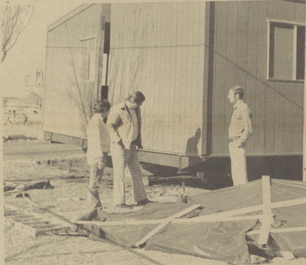
TEACHERS BROUGHT their classes to observe and staff spent their lunch breaks watching two halves of a modular unit join to form a new Skills Center at the Warm Springs Grade School. Located next to the library, the unit will house math and reading resources, provide a place for individualized instruction, and serve as head-
