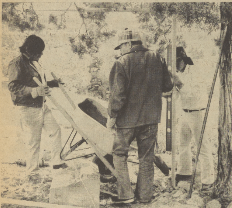
SHOWN IMBEDDING fence posts in cement are Gerald Charley (left), Lloyd Eder, and Delson Suppah, right. The workers should be finished at the Tenino Site this month.
