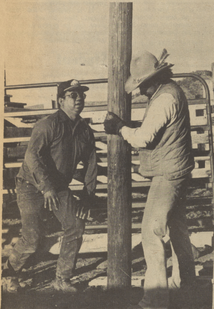
MEMBERS OF THE WARM SPRINGS RODEO Association are working on badly damaged holding pens behind the chutes under the direction of repair forman Levi Kennedy, also pictured is Evans Spino, assistant.
