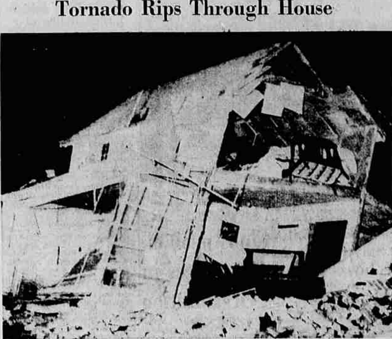
HIGH POINT, N.C.—This house was torn in half by a tornado that hit the western edge of High Point Friday night. A neighbor rescued Mrs. H. L. Shelton, 34 and her 18 months old granddaughter, who were alone in the house, from the debris. Neither was seriously injured. The baby apparently slept through the storm. (AP Wirephoto)
