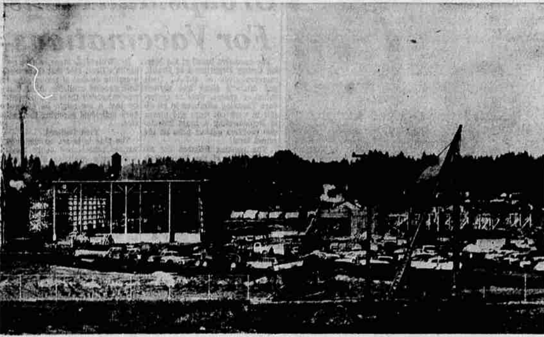
One of the largest industrial plants now rising in Oregon is the Georgia-Pacific pulp mill at Toledo, pictured above. The plant is to cost $40,000,000 and will be completed in 1958. About 150 men are now working on the job with 1,000 planned at the peak of construction. (Capital Journal Photo).
