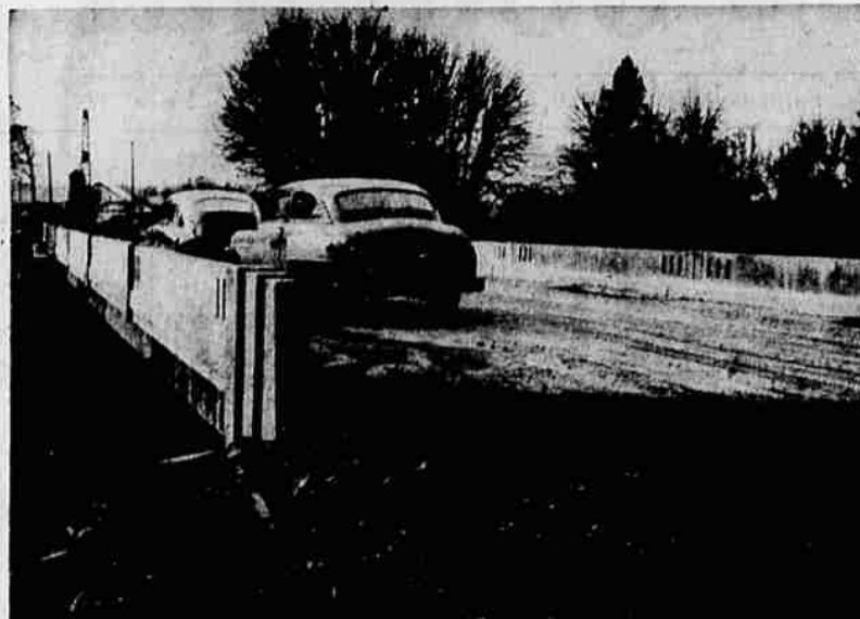
Only painting, dependent upon good weather, remains to complete new Marion county bridge spanning Champeog creek, opened for traffic Feb. 5. This reinforced concrete structure, supported by nine bents of piling, has a total length of 200 feet and a 26-foot roadway. United Builders of Beaverton erected the structure.
