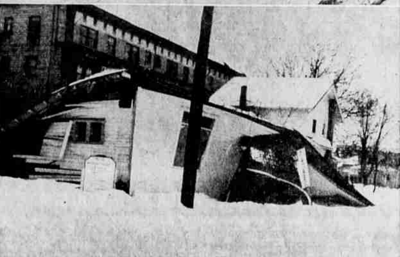
Downtown marquees were not designed to carry 27 inches of heavy, wet snow and many collapsed as did this one on the Court street side of Millers store. Center: Snow on the night of January 31, 1937, crashed this large range of greenhouses on Market St. Lower: Churches also suffered in heaviest snowfall ever recorded in Salem. Shown is wreckage of the Christian Missionary Alliance tabernacle on Ferry St.
