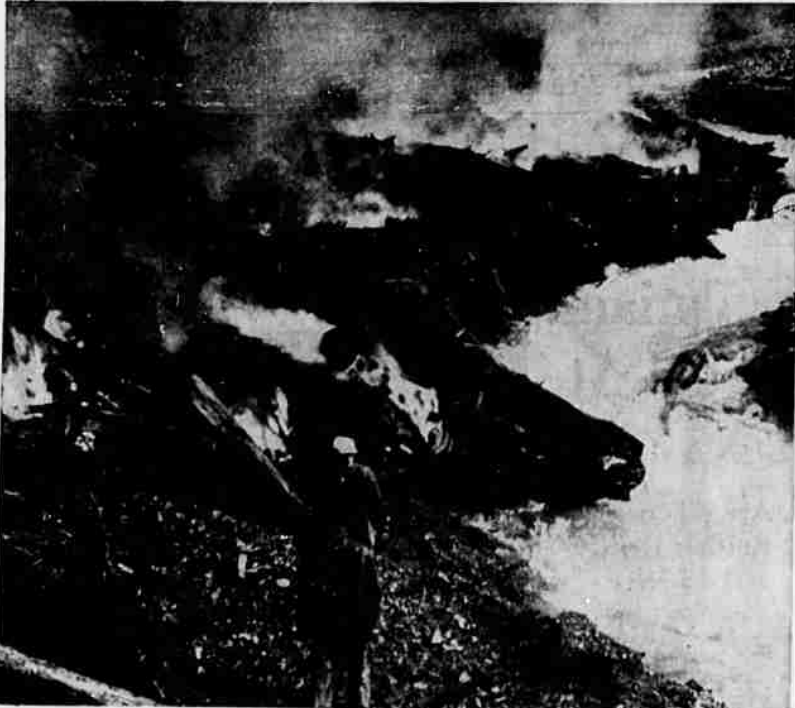
A crew of 25 men working under the state highway department supervision are shown piling and burning drift wood and debris from logging operations carried by flash flood down Sardine Creek to form a dam where the stream passes beneath North Santiam highway. At this point the stream backed up, overflowed the highway with drift, and carried away sections of guard rail. (Capital Journal photo).
