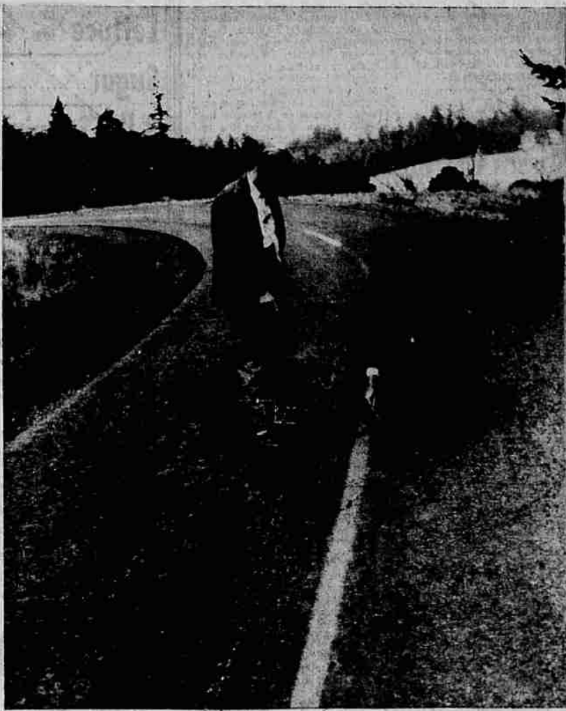
Marion County Engineer John Anderson, standing, and Commissioner Roy Rice point out cracks in 33-year-old pavement on Macleay road at a point where resurfacing and realignment of curves need attention. County court members took a 140-mile tour Wednesday to see where they could spend $875,000 in federal funds, decided they could use a lot more. (Capital Journal Photo)
