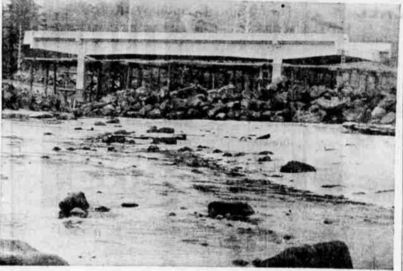
Top view shows expanded vista from a 4.16 mile section of new construction that takes Oregon's coast highway 101 over and above Otter Crest by easy grades and wide curves. Shown below in this photograph is a portion of the old narrow and crooked road. Beyond on a point, is West Shore manor. Center view shows a new and spacious parking area overlooking the Pacific and Otter Crest. Reconstructed highway around Otter Crest will be open for public usage by September 15. Cost of the project will be $1,600,000. Below is a view of a new structure over Fogarty creek where a state park is now under construction. Realignment and reconstruction of highway 101 is being accomplished between Depoe Bay and Miner creek to the southward.
